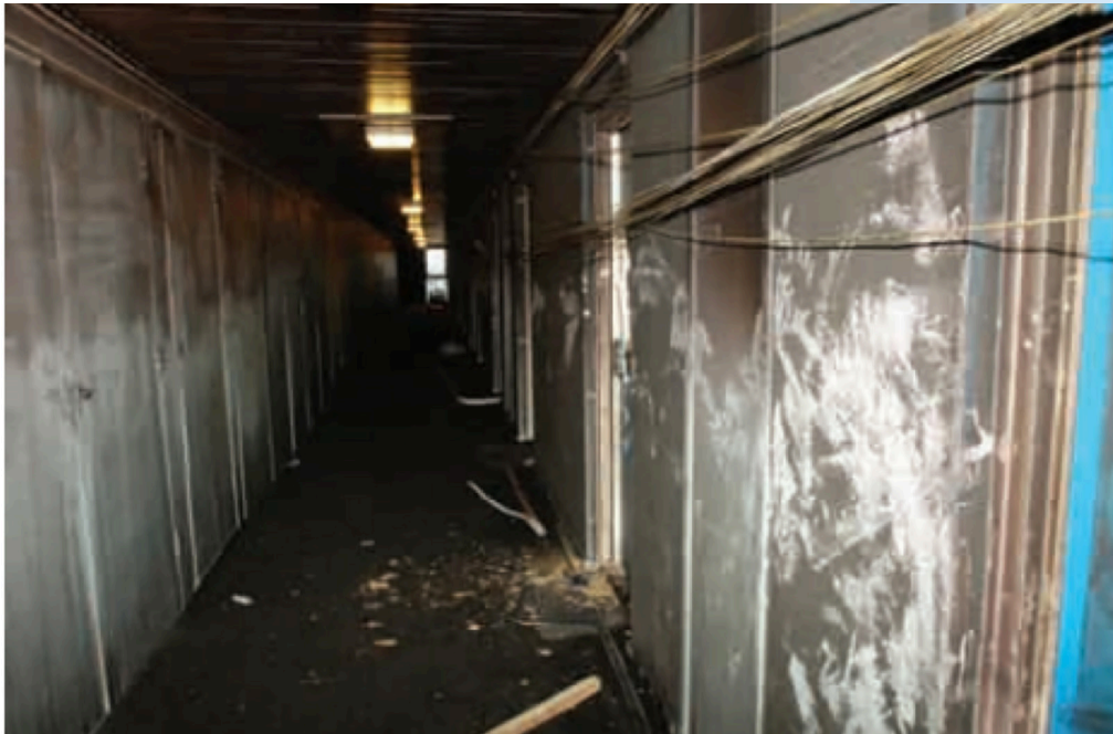
Post incident photograph showing conditions on the eleventh floor after the escape door from Flat 27 was left open, Note the displaced cables.
